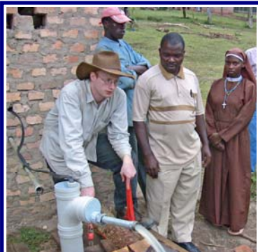
Les tests the solar pump after it has been installed in the completed well
