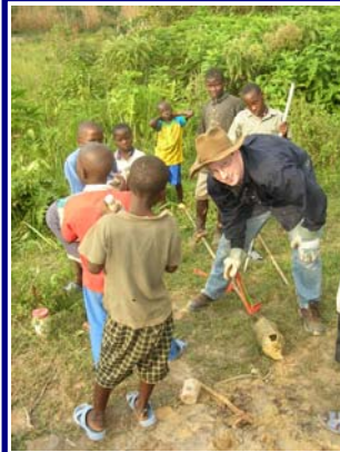
Les extending the handle on the auger in order to deepen the pilot well
