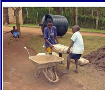
Schoolboys haul cement to build a foundation for the roof rainwater catchment tank
