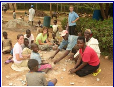
Melissa, Christa, and Holli help break rock into smaller aggregate for the sand bio-filter
