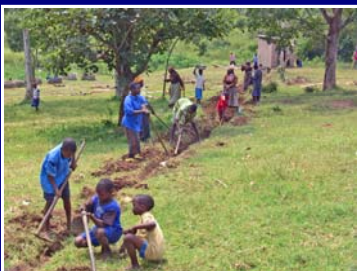
Students and staff digging a trench for the underground solar power cable
