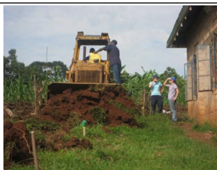
A contractor was hired to level the land for phase one and future construction. Christa and Dabney are inspecting the work. It was a great experience keeping the contractor on task.
