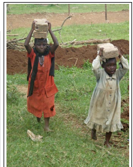
Girls help transport bricks to the construction site. The dorm will be their new home.
