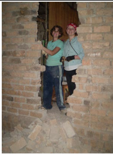
Christa and Tara knock a hole in the wall for a new door as part of the renovation and expansion of the medical clinic. Space will be more than doubled and two triple-decker beds will be installed to accommodate children when they are sick.
