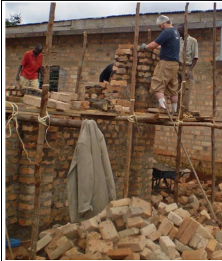
Tomas, other team members, and local volunteers constructed the brick walls. The scaffolding is tied together with twine. The bricks were formed and fired by the staff and children from clay on the orphanage property.
