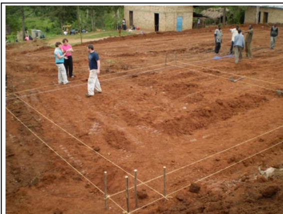
After the area was leveled Tara, Christa, and Tomas lay out the footings for phase one construction.
