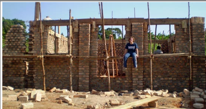
The structure is complete except for the roof which will be constructed by a contractor. Notice the reinforced concrete ring beam at the top of the walls.
