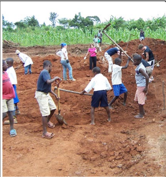
Everyone pitched in to do the final leveling and to dig trenches for the footings. The footings were constructed of brick to a depth of three feet.
